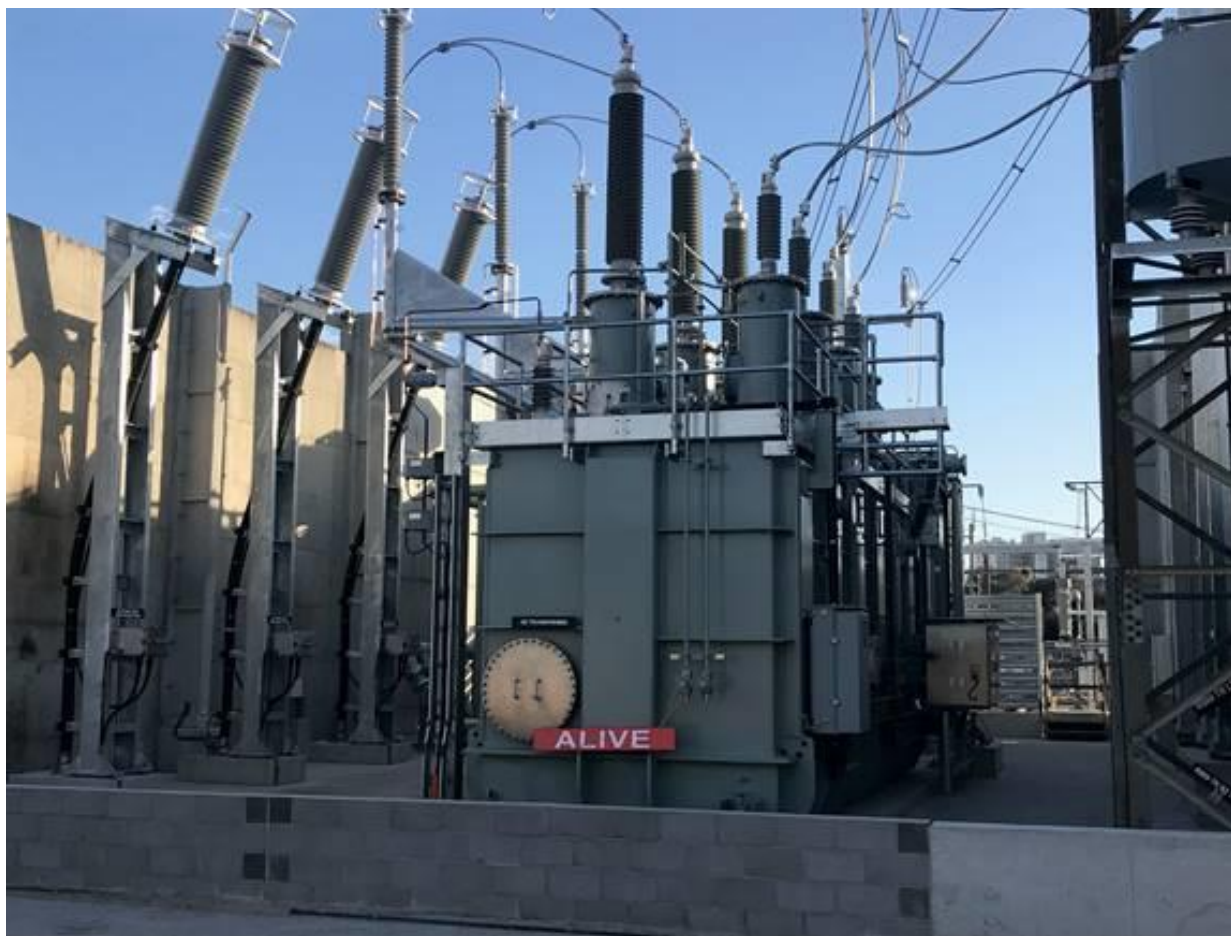
West Melbourne Terminal Station B3 220/66kV Transformer (Image credit: AusNet Services)
